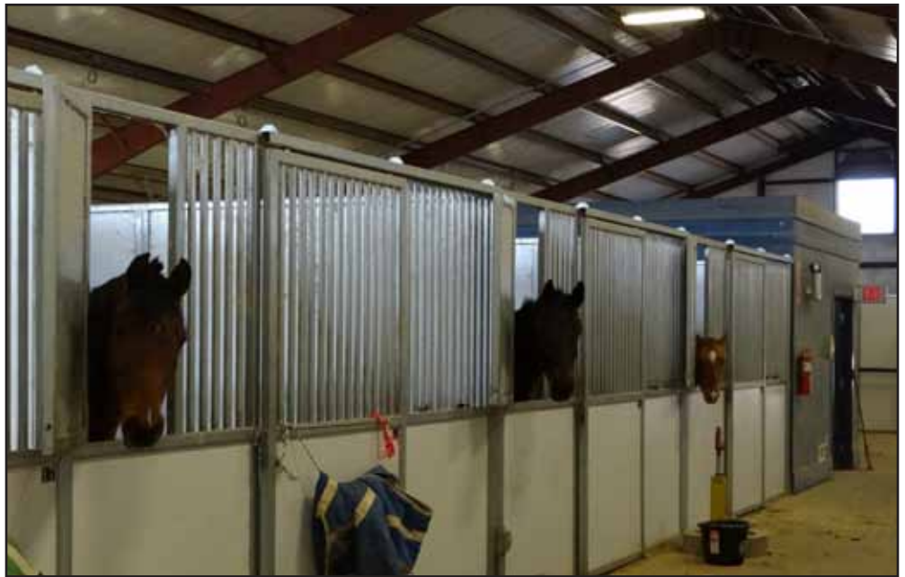
This depicts a well-designed barn. Stalls are made of pipe and fire retardant materials, electrical systems are in conduit (along the ceiling), aisles are wide and clear, exits are clearly marked, and there are fire extinguishers strategically placed throughout. Photo courtesy of Klaire Tardiff
